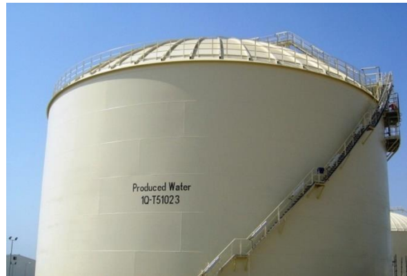
Produced water storage tank 4
